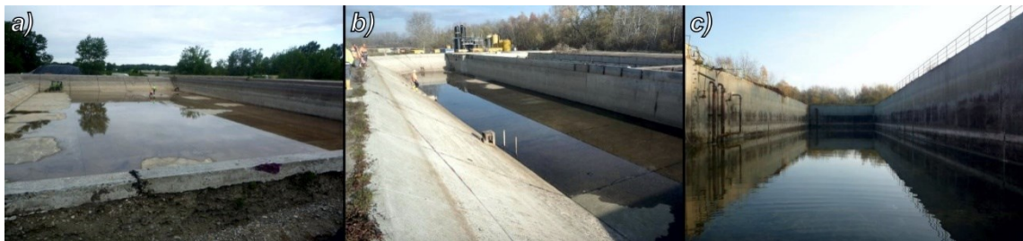
Fig. 6.4: Basins (a: sub-basin A of the basin compound ABC, b: basin D of the basin compound DEF, c: Basin H), which may serve for re-use as seasonal thermal energy storage at the IN-Campus (cf. FIG. 1.4).
